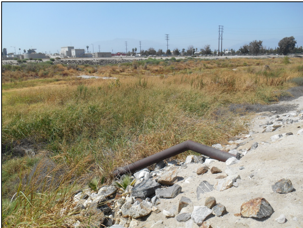
Photo 4 – Looking northwest at Thorne 12 well blow-off piping towards Flood Control Twin Creek channel and W Orange Show Road.
